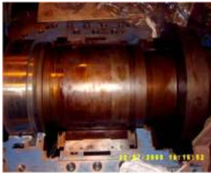
Thrust bearings without purification systems installed
